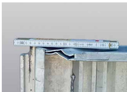
Stair Tower ■ deformation / damage at one point of the frame profile on the landing guardrail
