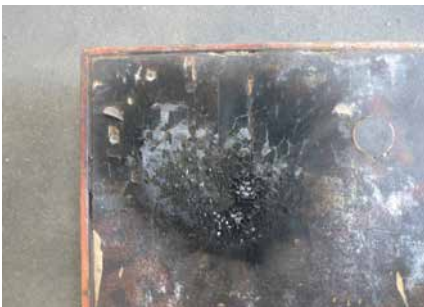
Damage caused by the effects of heat ■ Sheet replaced
