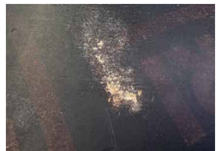
Damaged caused by the use of a concrete vibrator
