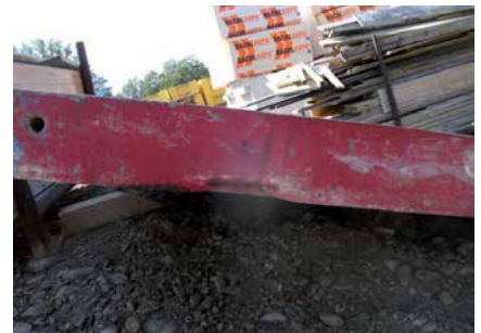
Damage to end profile due to incorrect use of the crane hook
