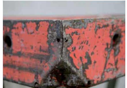
Crack in the welding seam
