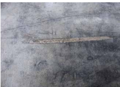
Damage > 1 mm deep
