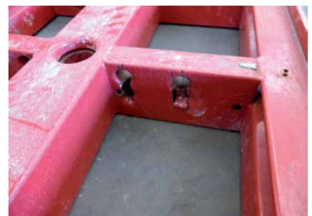
Sleeves of the perforated strut torn out
