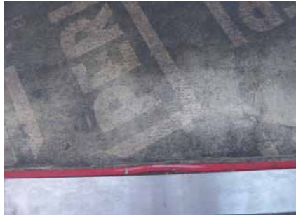
Bent formlining support > 3 mm
